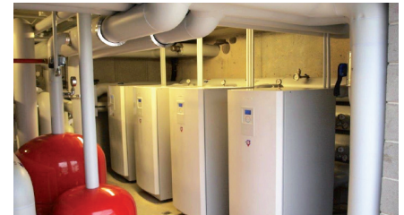
The heating room with Thermia Robust ground source heat pumps
